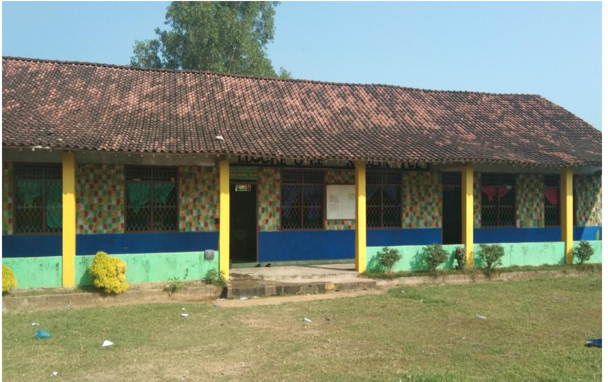
The condition of the Classroom
